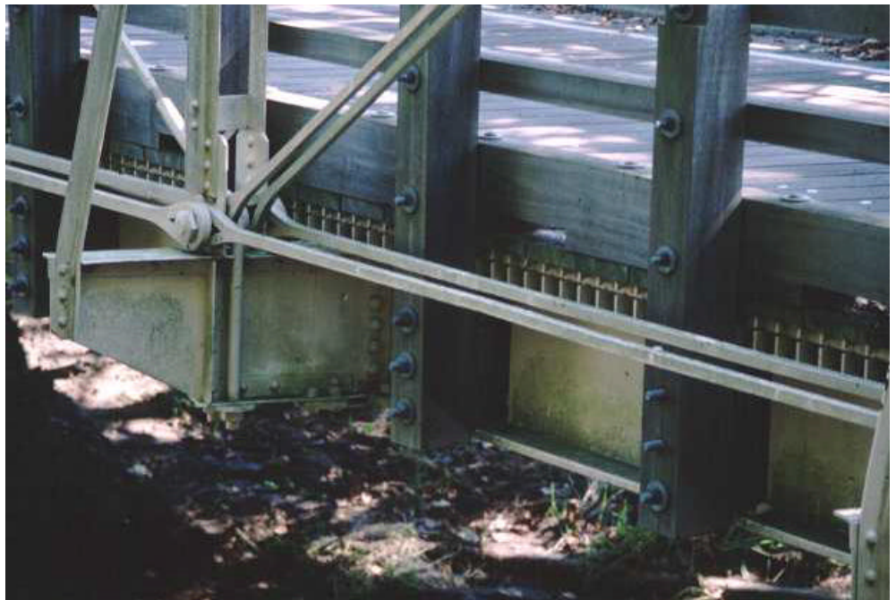
The restoration of the Wollaston Rd. Bridge involved dismantling the old bridge, building a new modern supporting structure, and rebuilding the old bridge on top of it.
