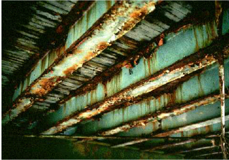
A glimpse underneath the Landenberg Bridge shows the consequences of the neglect the bridge has suffered.
