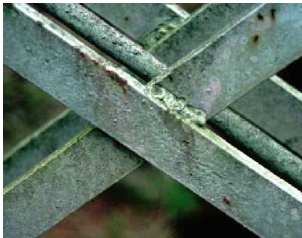
In a botched repair, the truss struts were welded together consequently weakening the entire bridge.
